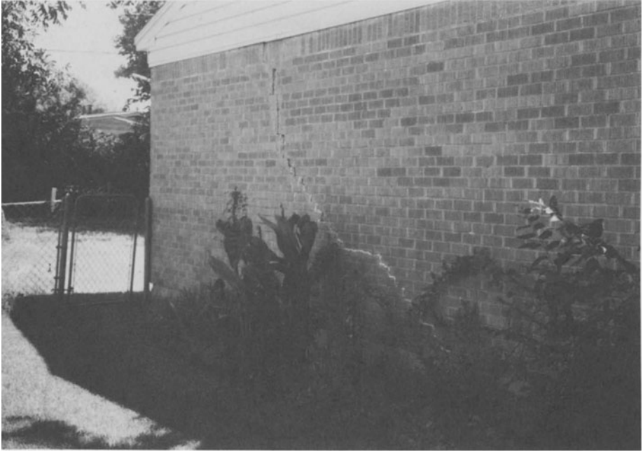
FIGURE 11-9. Damage to a residence, caused by differential settlement.
