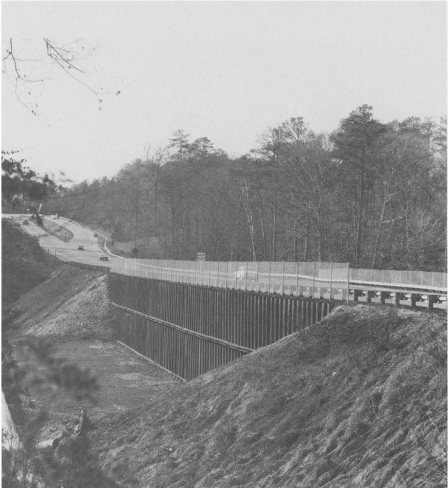
FIGURE 8-4. Bethlehem PZ27 sheet piling stabilizes this busy roadway in a marshy location near Williamsburg, Va. [Ref. 3]
